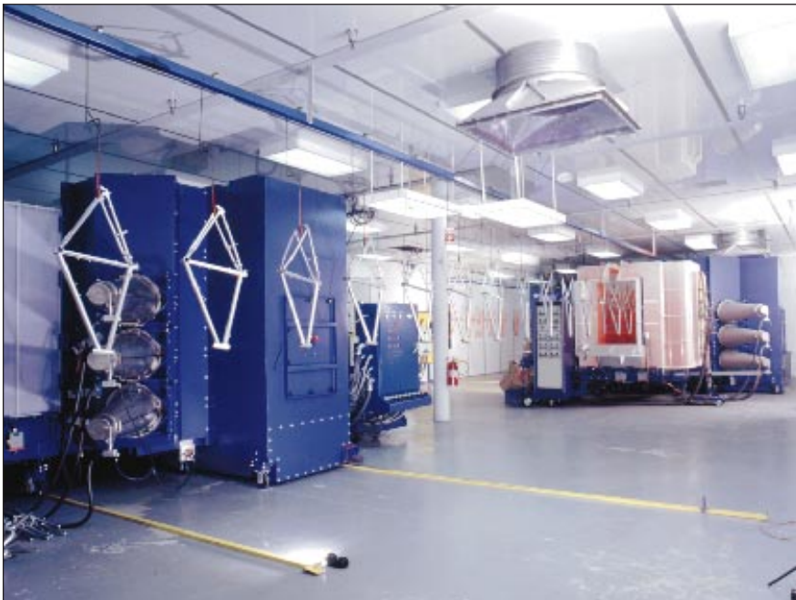
The roll-on/roll-off Nordson Cyclo-Kinetic booths allow color to be changed off-line without stopping production. (Photos courtesy of Nordson)
